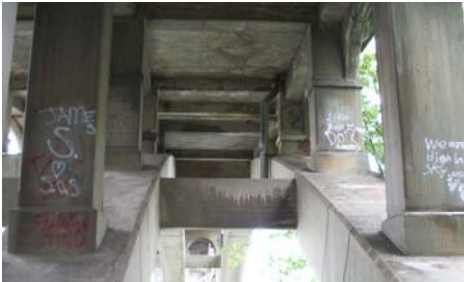
Figure 8 Graffiti on columns underneath bridge
