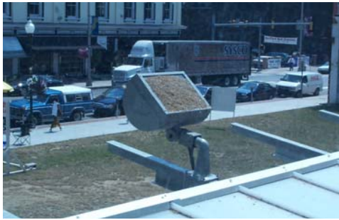
Figure 25 Light fixtures need to be cleaned periodically, or else...
