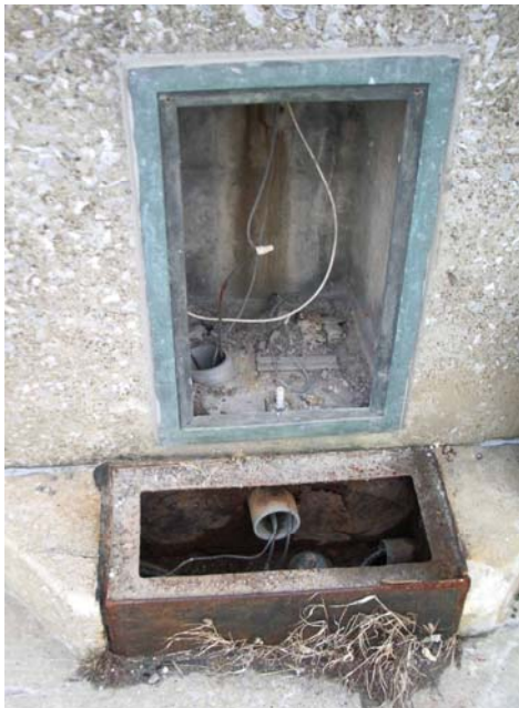
Figure 10 Electrical junction boxes at base of a light pier
